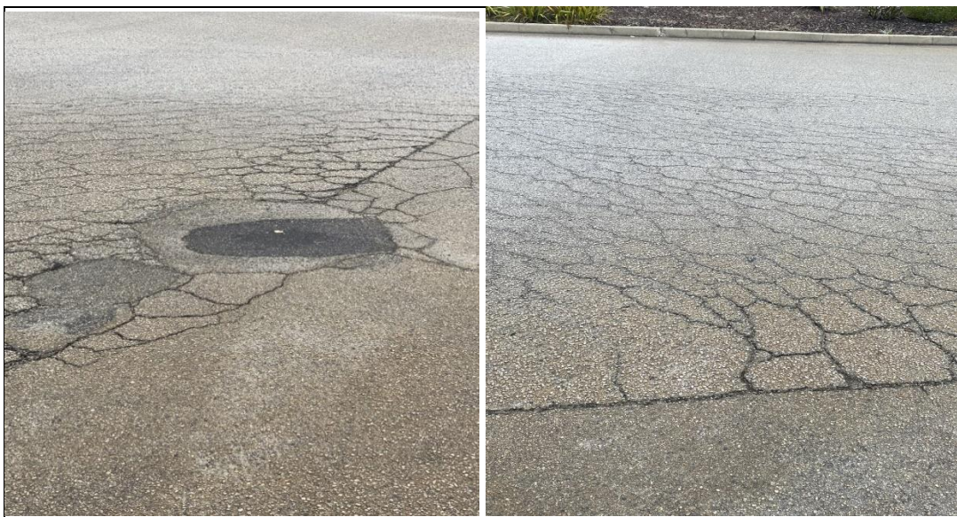
Figure 5.1: Pavement deformation and cracking (photos by Nuha)
