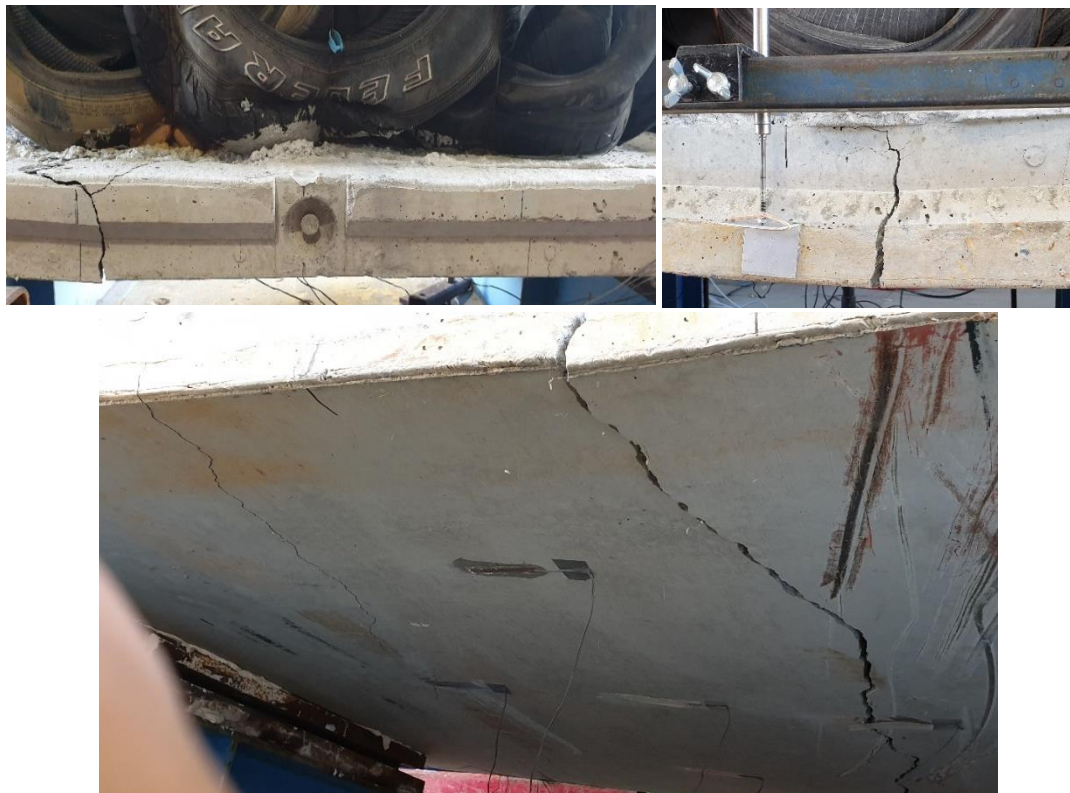
Figure 3-8 Crack pattern in bottom concrete wall during experimental testing
