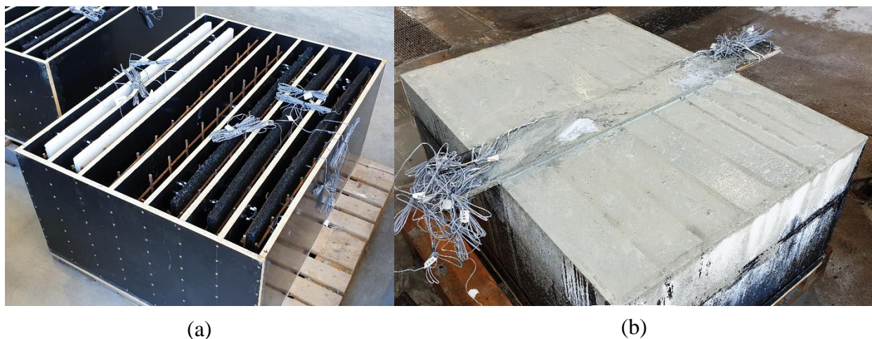
Figure 4-7 (a) Timber formwork and location of core material (b) Final finish after pouring SCC
