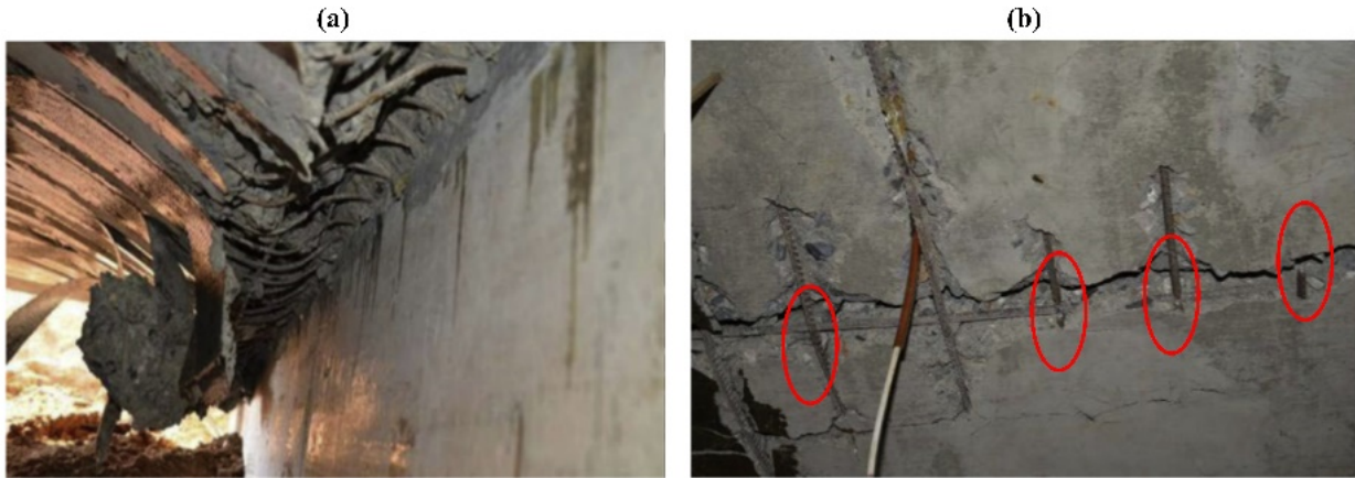
465 466 Figure 15. The bending and tensile failures of reinforcement (Chen, et al., 2015). (a) bending failure, and (b) tensile 467 failure.
