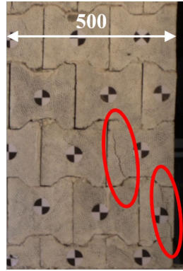
b) Right toe cracking at 40mm lateral displacement
