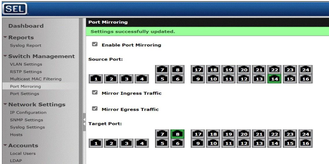
Fig. 6.6. SEL Ports Connected To Test Kits, IEDs, MU And Laptop For GOOSE and SV Traffic Flow Conditions.
