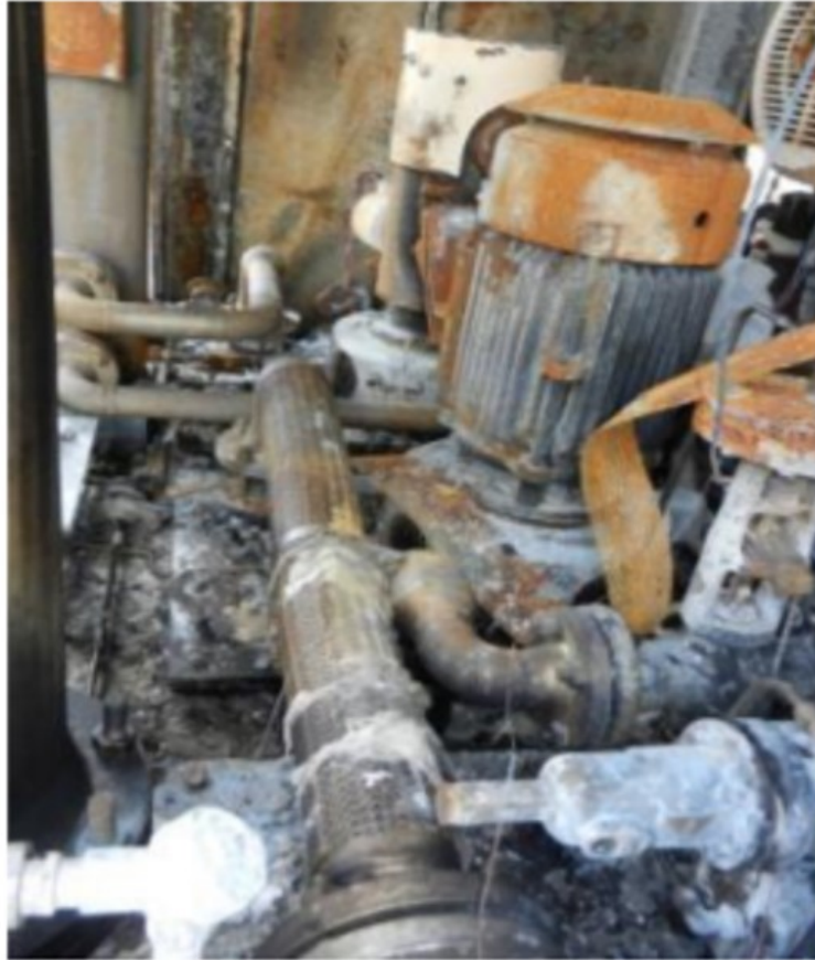
Figure 3.16: Fire incident due to dry gas seal failure
