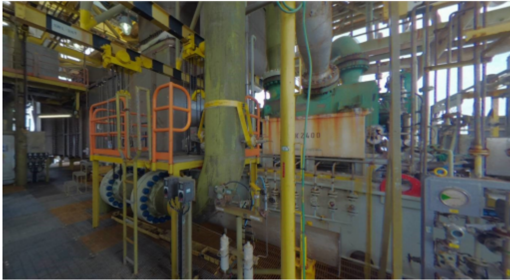
Figure 3.3: Compressor in offshore compression platform
