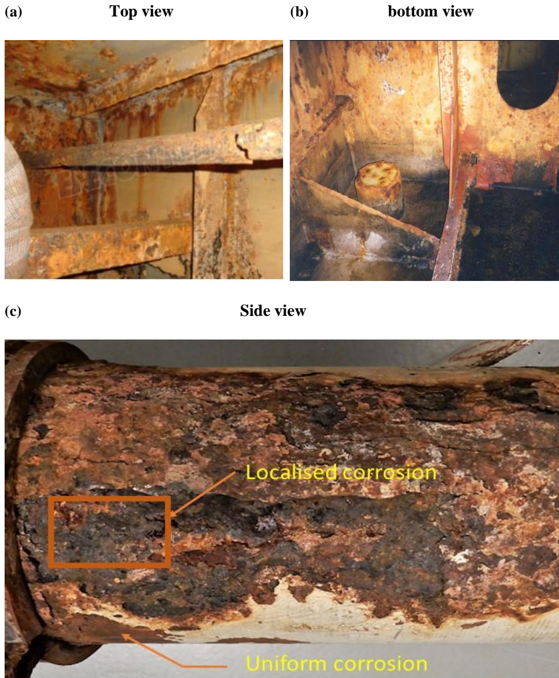
Figure 2-2: Corrosion of carbon steel in enclosed environments; (a-b) inside a ballast water tank used to stabilise a ship [52] (c) under insulation [53].
