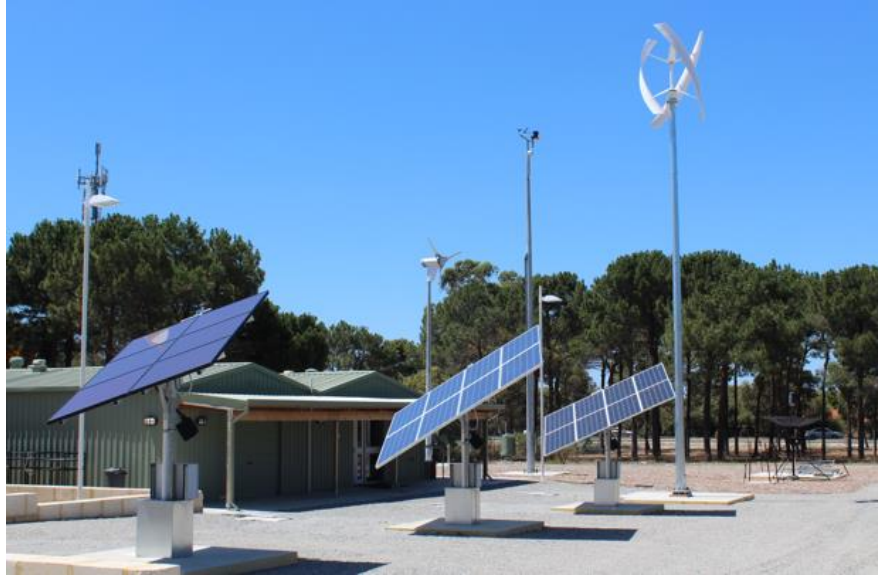
Figure 3.2 Green Electric Energy Park at Curtin University (Image credits: Prof.Sumedha Rajakaruna, Director Green Electric Energy Park)
