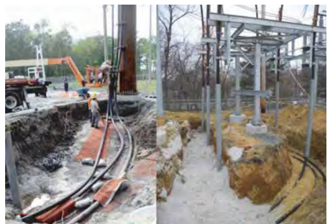
Figure 28 Direct buried section near a compact transition pole with one cable per phase (left) and conventional risers with two cable per phase (right) [31]
