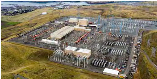
Figure 35. HVDC Converter Station (ABB 17 )
