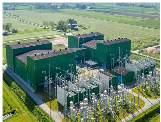
Figure 32. HVDC Converter Station (Hitachi Energy [27])
