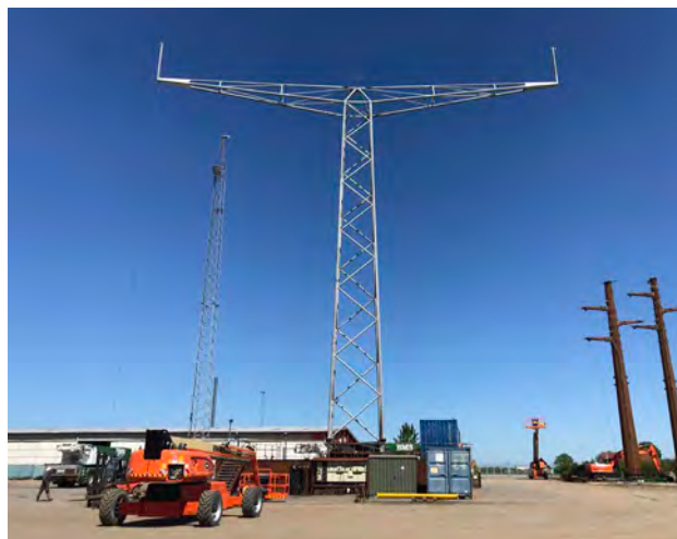
Figure 14. 400kV Double Circuit Thor-gi Tubular Steel Structures (Energinet)
