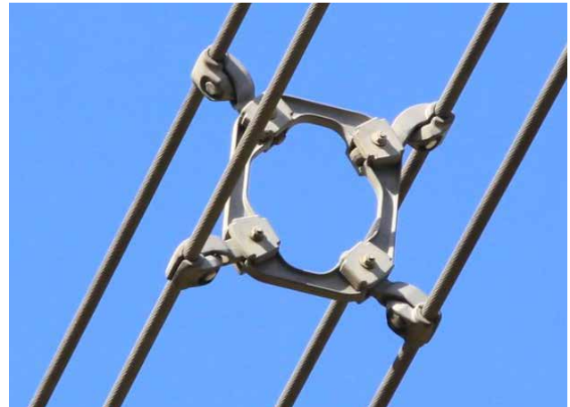
Figure 2. Transmission Line Quad Bundled Conductor with Spacer (Marcus Wong)
