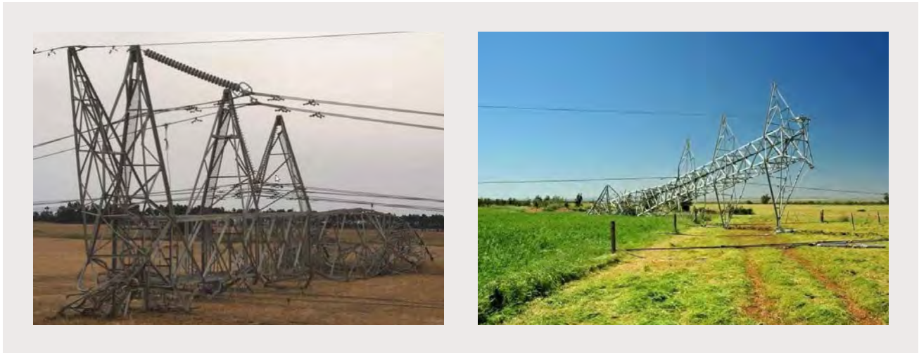
Figure 9. Fallen 500kV Double Circuit Tower, Victoria (Zinfra Pty Ltd.) and 275kV tower, South Australia (ABC News: Dean Faulkner)
