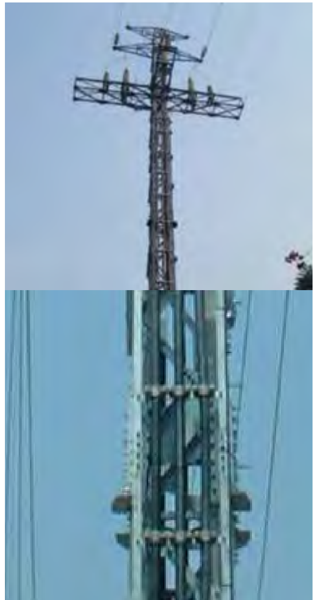
Figure 30 Junction tower with structural steel (left) and lateral view of flat arrangement of cables (right) [50]
