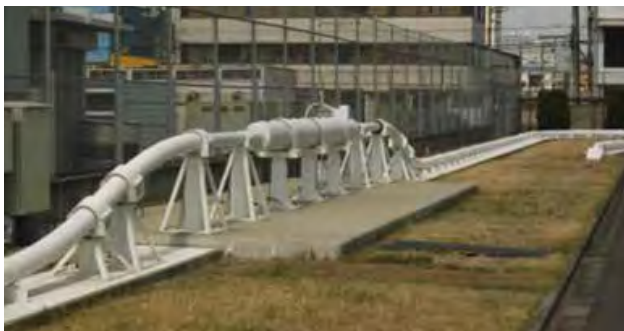
Figure 24 TEPCO AC HTS cable with a joint at Asahi substation in Yokohama/Japan [52]
