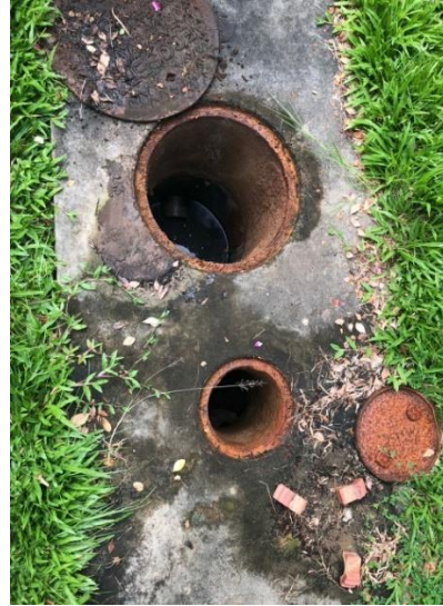
Figure 3.3: Excessive septic sludge.
