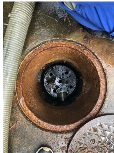
Figure 3.5: Empty septic tank after desludging.
