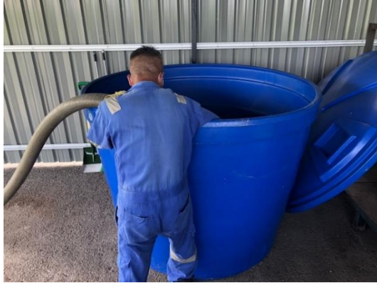
Figure 3.6: Transferring the septage into a storage tank.
