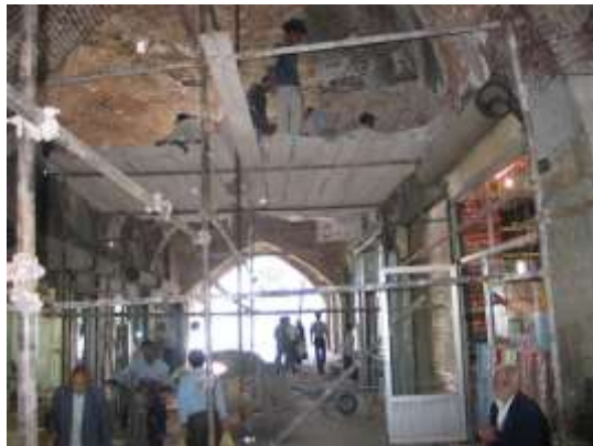
Figure 7.6: A restoration workshop while the flow of people passing below and continue the daily life. Photograph by Shahin Tolouashtiany 2000.
